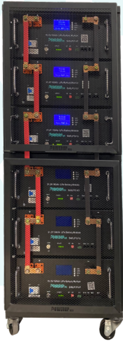
SIX BATTERY RACKS
